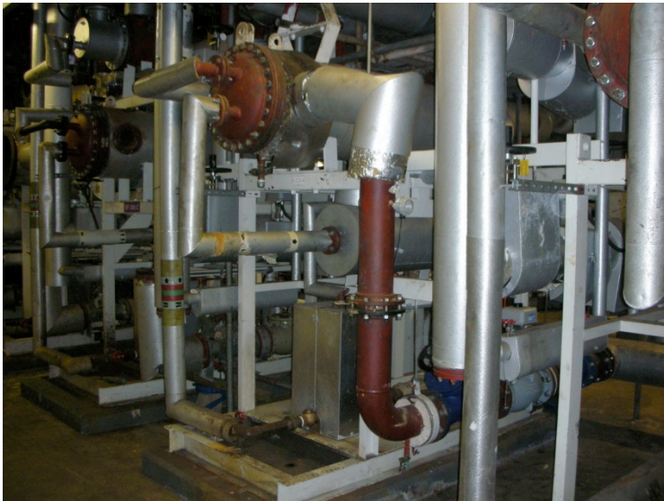
Figure A1.2 – missing thermal insulation
