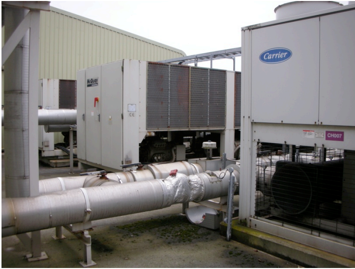
Figure A1.1 – chiller compound
